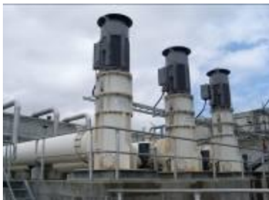
Bearings for Pumps
